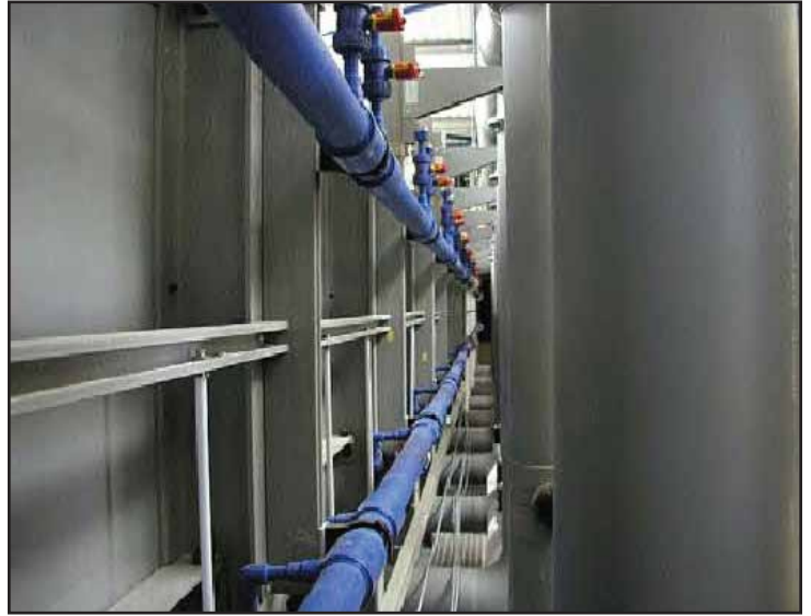
AGRUAIR PE compressed air piping installed at a chemical plant
